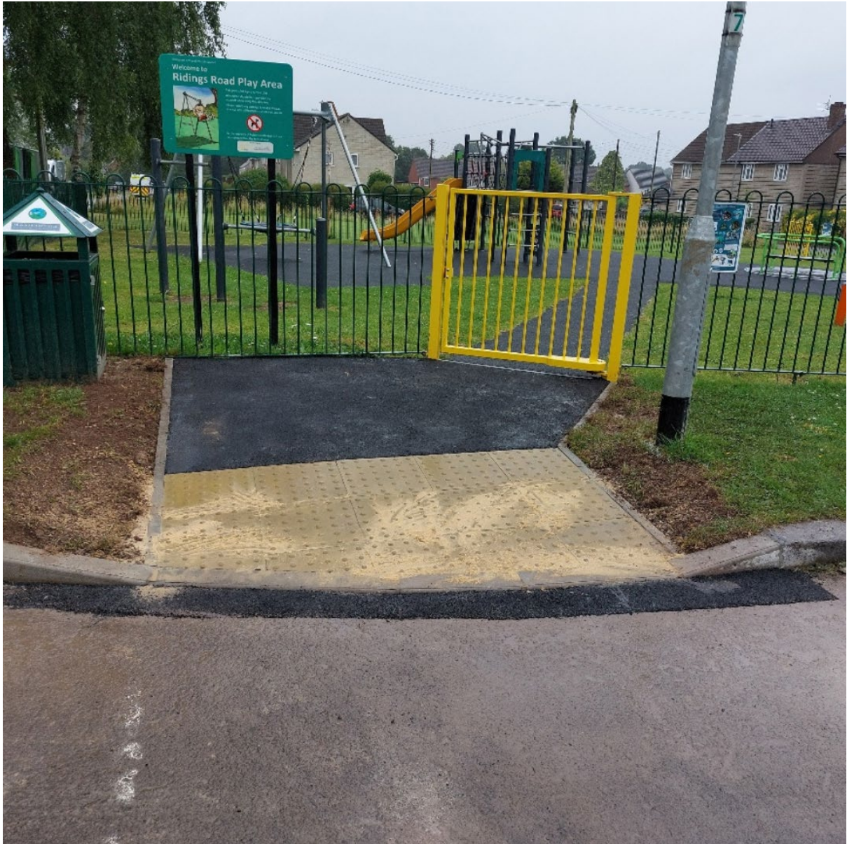
Figure 26: Newly installed drop kerb on the pavement outside of the entrance gate of Ridings Road Play Area
